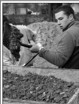
Airman 1st Class Jeremy Sealey from the 422nd Communications Squadron shovels dirt and gravel onto a loader to be used on sidewalks.
